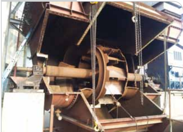
Original forward-curved, radial-tipped fans.
